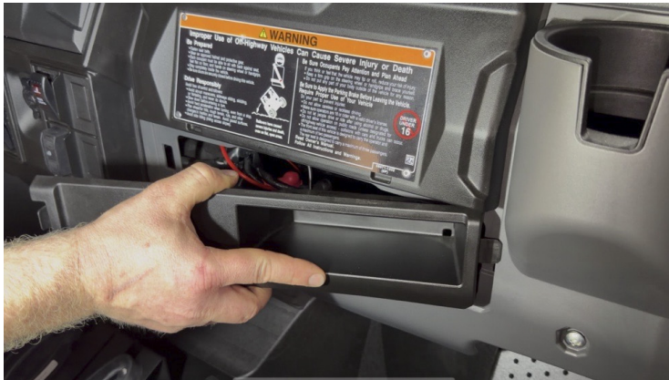
FIG 21 - Route the pod light pigtails to the lights and plug in the lights
