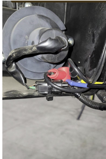
FIG 27 & FIG 28 - Fasten Contactor Winch wires and Winch Extension wires to Junction Block
