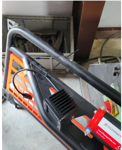
FIG 17 - Zip Tie Cube Light wire pigtail to Headache Rack
