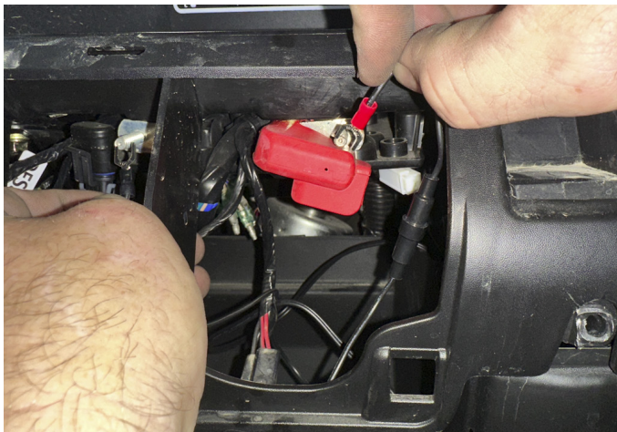
FIG 9 - Gain access to bus bar and remove OEM nuts in preparation for wiring
